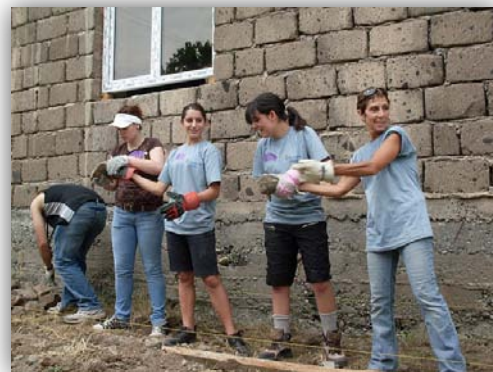
Team members pass stones to each other to lay the concrete apron that guides water away from the foundation.
